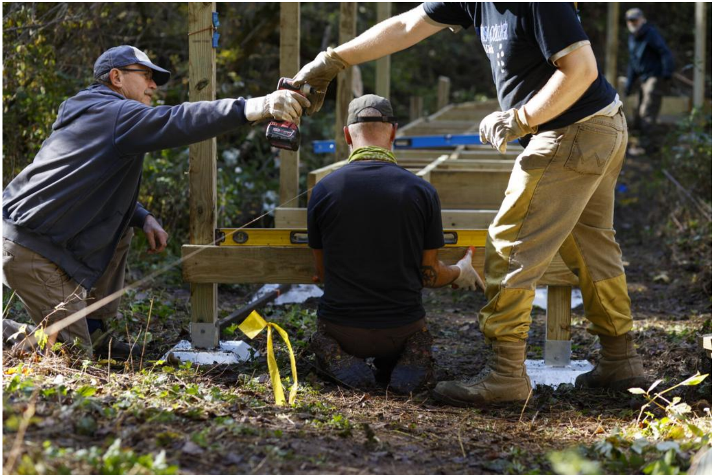
Gary Krause, of Weston, Craig Johnson, of Madison, and Michael “Moose” Moen, of Middleton, help build 92 feet of boardwalk on a new segment of the Ice Age Trail in Cross Plains.
