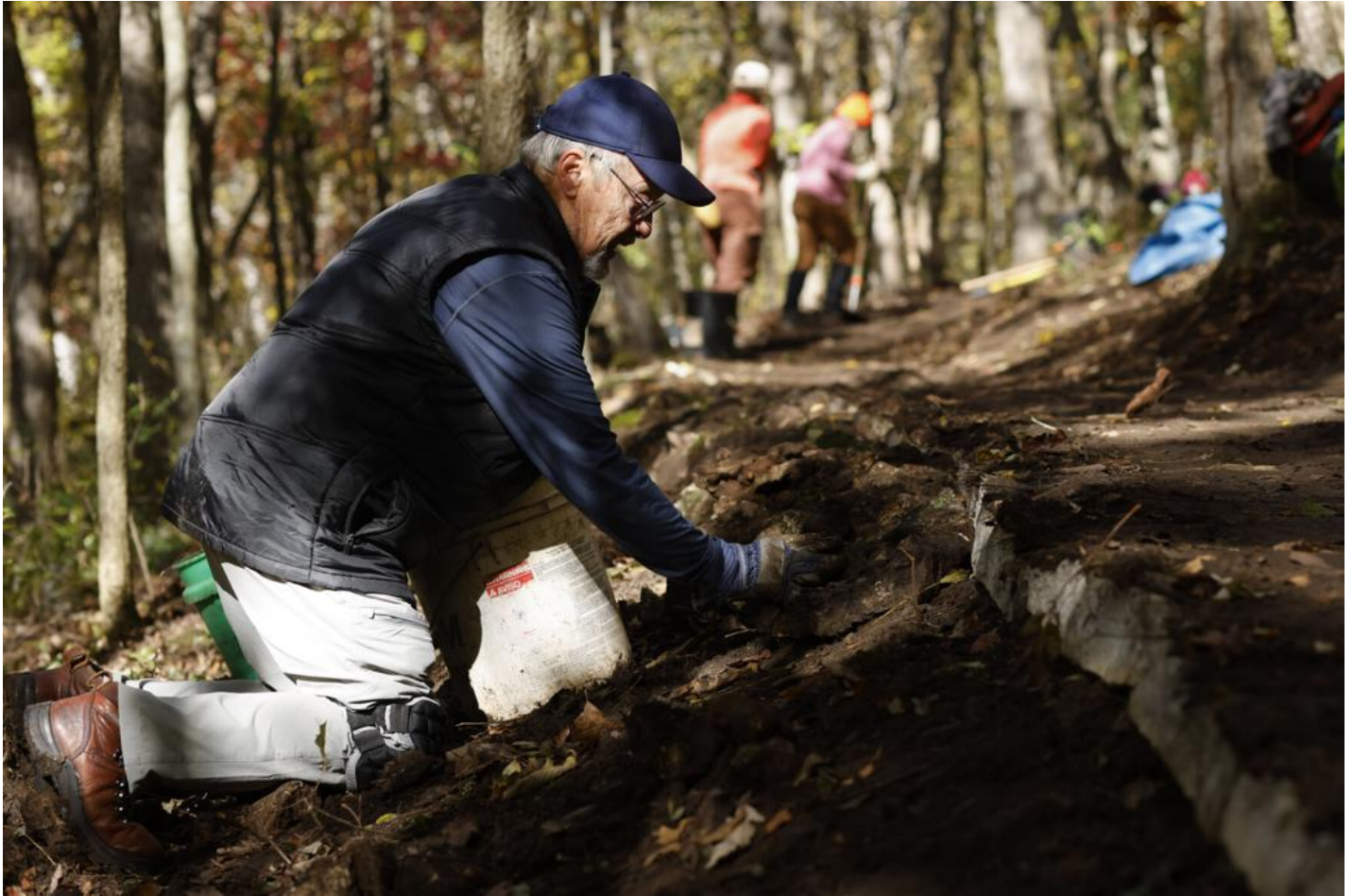
Wayne Surguy, of Cedarburg, WI places stones to act as a retaining wall on new segment of the Ice Age Trail in Cross Plains.
