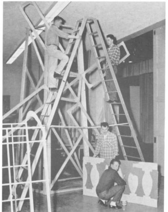
The construction of the mill posed many problems which the stage crew had to overcome. Shown here are Tom Lake and Bradley Paulson.
